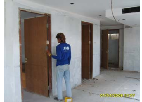
Picture 36: Wooden door frame and
