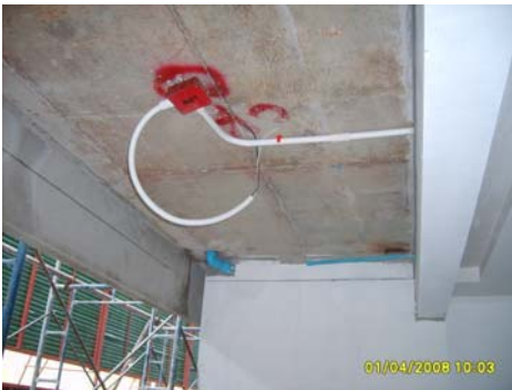
Picture 22: Duct and Wiring system at
