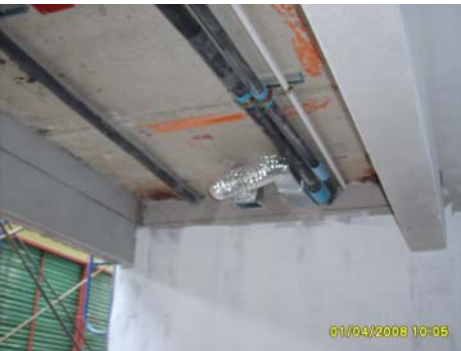
Picture 26: Duct and Wiring system at
