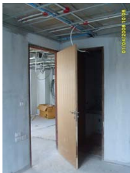
Picture 41: Wooden door frame and
