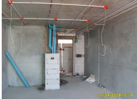
Picture 70: Duck piping and wiring
