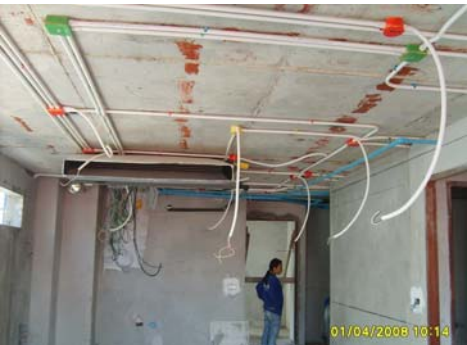
Picture 51: Duct piping and wiring
