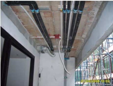
Picture 20: Duct and Wiring system at
